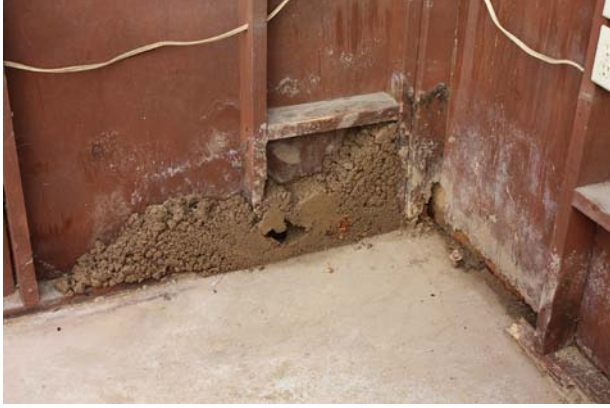
Photo 3: This third pile of dirt was smaller because plywood had been nailed to the studs.
